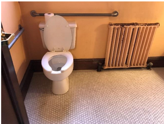
Typical Plumbing Fixtures
