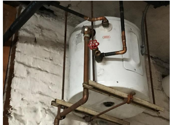
Hot Water Heater
