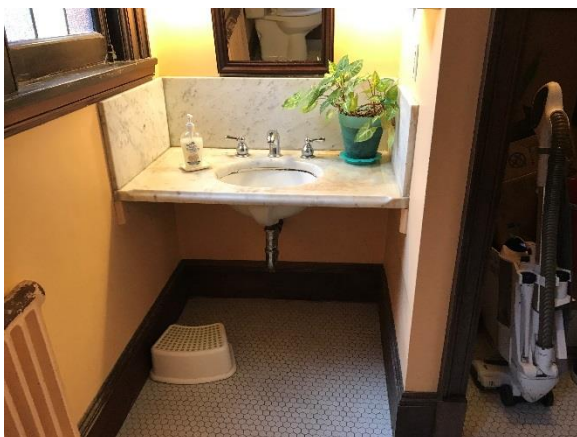
Typical Plumbing Fixtures
